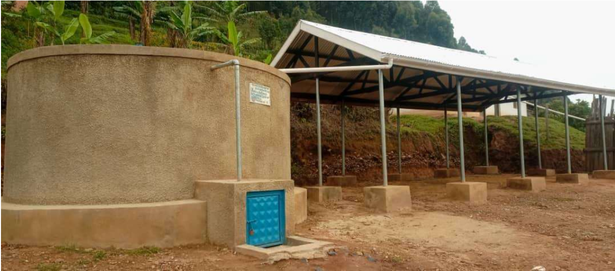
30m3 Rainwater Harvesting Tanks with a roof catchment
